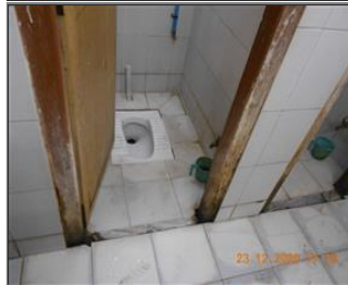
Photo of the sanitary facilities DSCN4719.jpg
