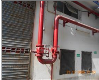
Photo of fire safety equipment DSCN4692.jpg
