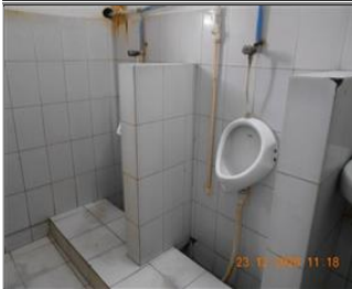
Photo of the sanitary facilities DSCN4718.jpg
