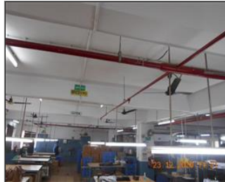
Photo of fire safety equipment DSCN4728.jpg
