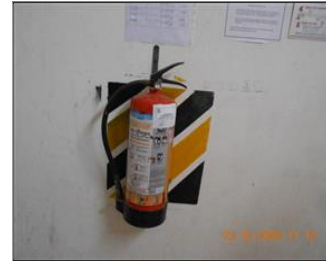
Photo of fire safety equipment DSCN4702.jpg
