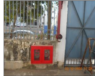
Photo of fire safety equipment DSCN4687.jpg
