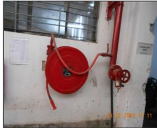
Photo of fire safety equipment DSCN4696.jpg
